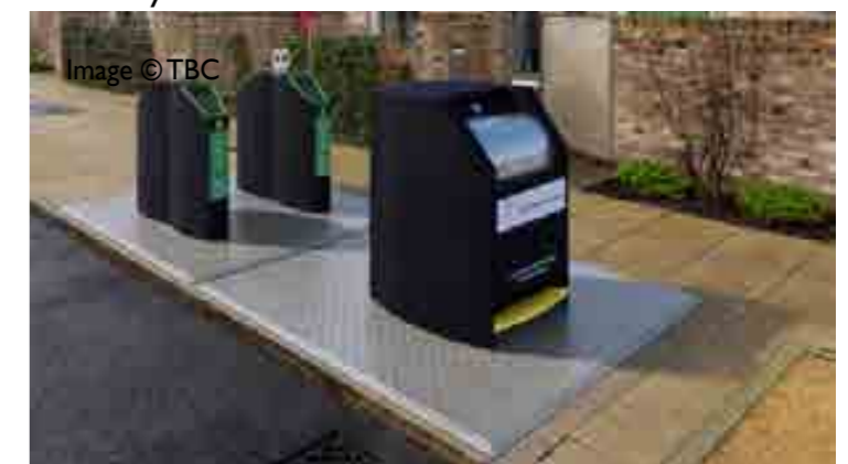
Image © TBC Underground refuse and recycling system
